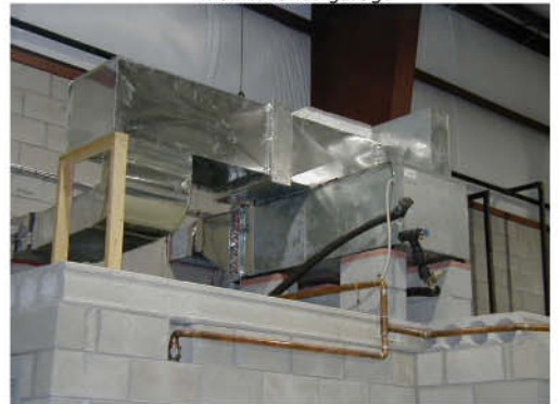
Offices geothermal heating and cooling unit, with 5 zones of control
