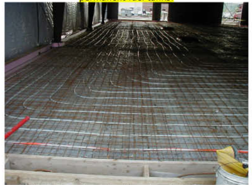
WIRSBO geothermal radiant heat in 6,000 sq.ft. maintenance garage
