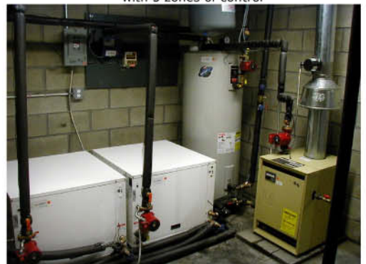
Boiler equipment room designed by Smart-Energy. Two WaterFurnace geothermal boilers, thermal storage tank, and gas Emergency Backup boiler, as well as all sequencing and automatic setback controls
