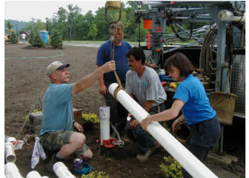
Sleeve installation by Jim Dwyer and crew, into one of the two 500 ft geothermal source wells. Now the permanent fuel tanks!
